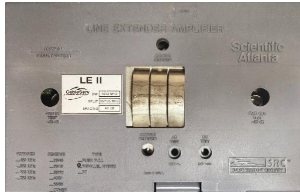
CableServ LEII/III 1 GHz Forward Upgrade
